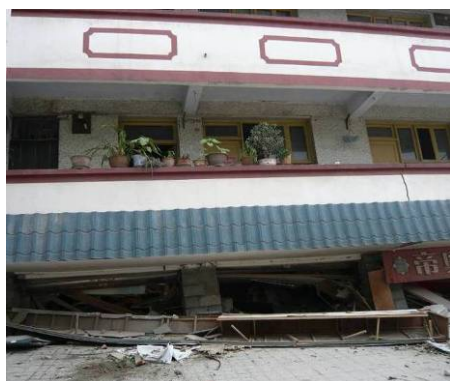
(c) 某底框住宅底层倒塌，二层花盆仍在原位 (c) First story collapsed with the flower pots on the second story intact
